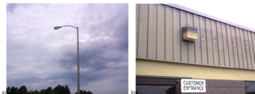
Figure 1: a) Sodium streetlight and b) sodium building light.
