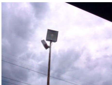
Figure 5: Mercury parking lot light.
